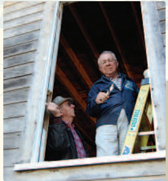
▶ Boutwells Landing residents Joe Carufel and Norm DuFresne repair the schoolhouse window frame.
